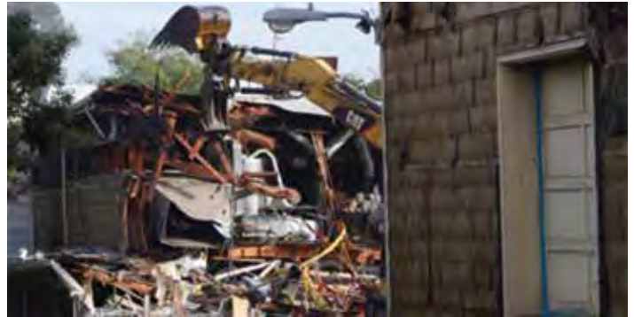
Demolition at the site of the USMS Officers' Training School, Alameda, CA. Photo provided by Carmen Reid.
