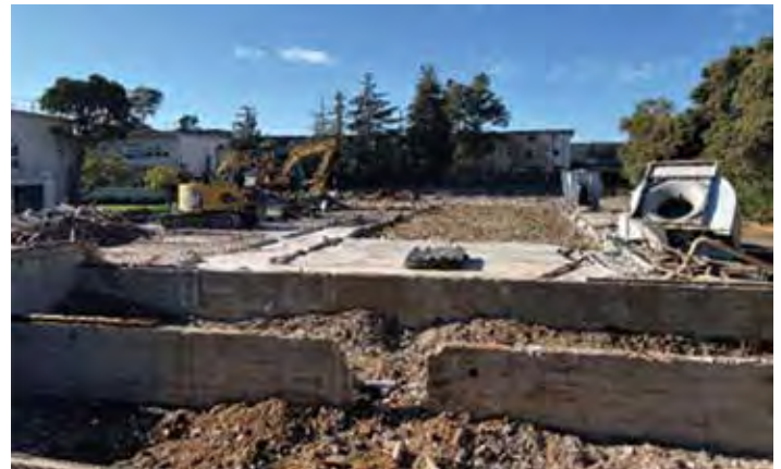
Cleared demolition debris at the USMS Officers' Training School, Alameda, CA. Photograph provided by Carmen Reid.
